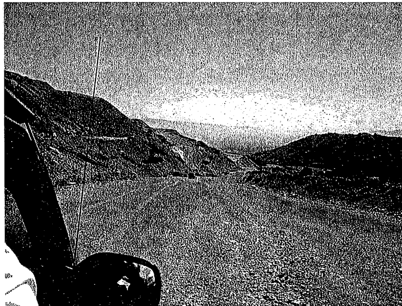
Photo 16: Rock check dams along main haul road on south side of WMSA to help control erosion, looking east. Dated August 25, 2011. Compare to 2010 inspection report photo 18.
